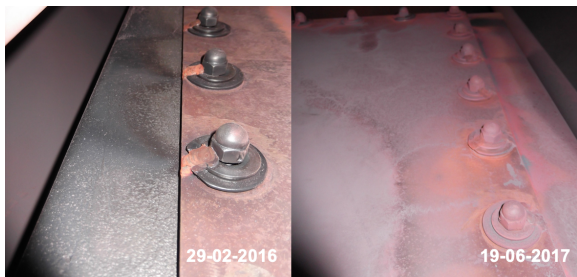
Figure 10: LP drum comparison (top of riser box)
